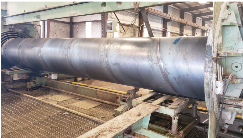
This newly formed steel cylinder with joint rings welded to each end has just been tested hydrostatically to make certain it is watertight.
