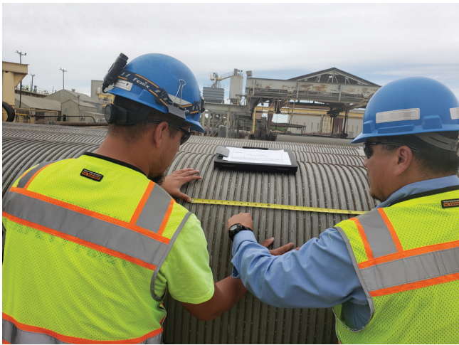
Quality control inspectors monitor wire spacing during prestressing operation. Prestressing wire is tested prior to wrapping and must be within limits specified in ASTM A648 and AWWA C301.
