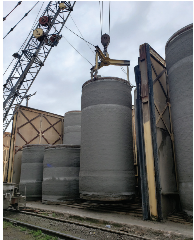
In the coating operation, a slurry of cement and water is sprayed onto the prestressing wire as the mortar is applied over the wire to form a rugged exterior wall that provides protection against corrosion.
