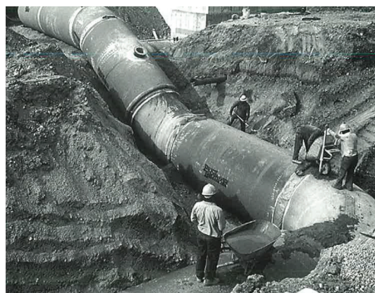
PCCP is ideally suited for many applications, such as this treatment plant. The precise custom fittings made this complex installation simpler to install with no field cutting or tapping.
