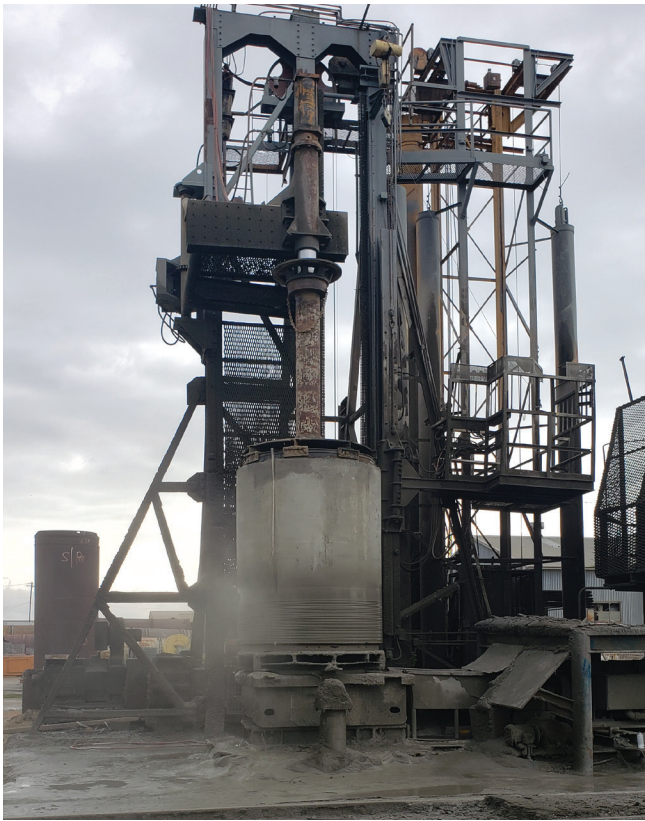
The concrete core is placed on the rotating platform of this vertical wrapping machine. Cement slurry is applied as steel prestressing wire is wrapped under tension around the core.
