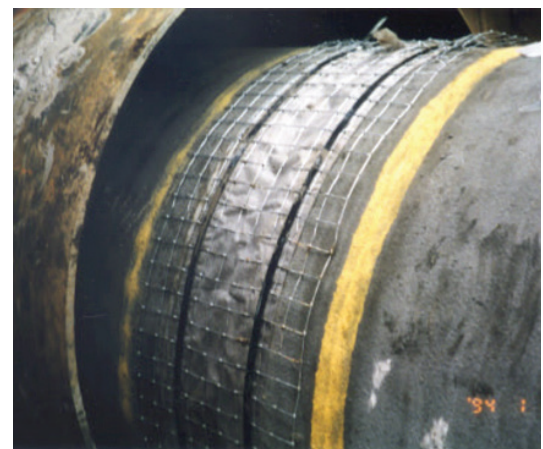
Figure 4: Light gauge steel mesh wrapped around the joint to support the wet grout in the grout band.
