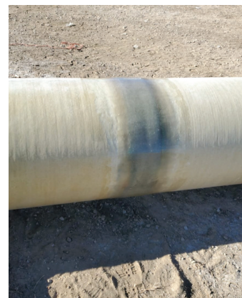
Joint lamination is similar to field welding steel pipes. FRP pipe joints are laminated with layers of fiberglass.
