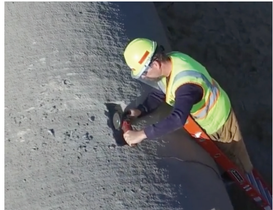
A Thompson Pipe Group worker cuts a dozen wires on a pressurized section of PCCP.
